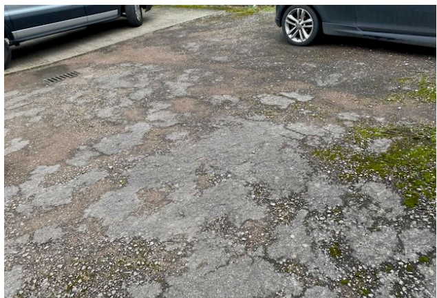
24. Tarmac parking space in poor condition.
