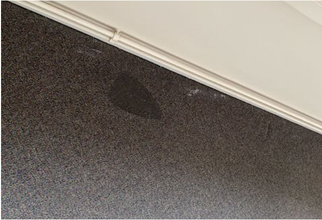
13: Worn/defective carpet to office on first floor.
