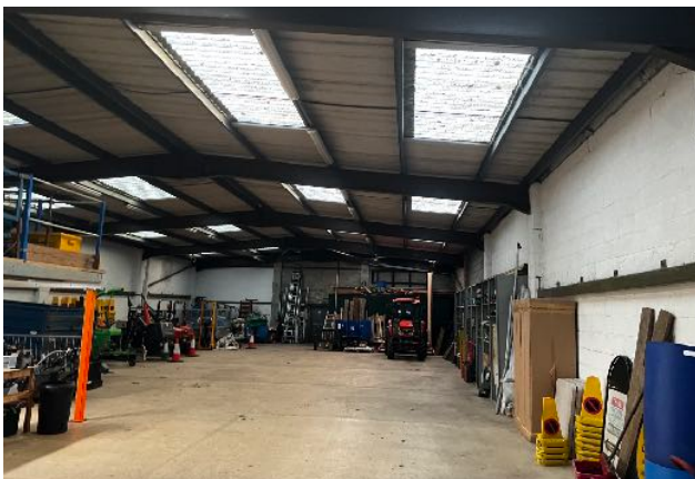
ME01 Warehouse lighting in need of replacement.
