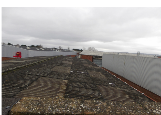
02: Lichen and Guano build up to coping stones.
