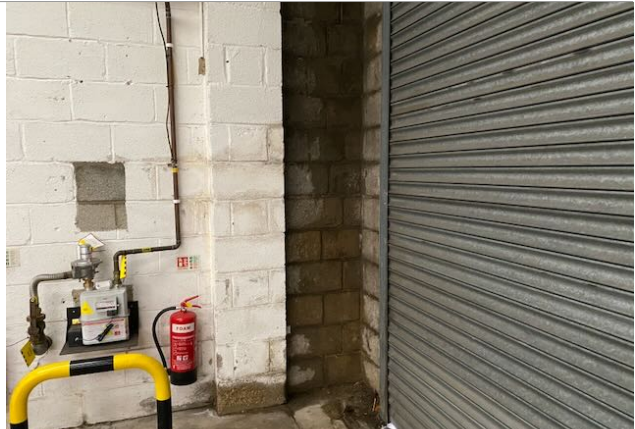
20. Saturated clockwork as a result of failed rainwater outlets.
