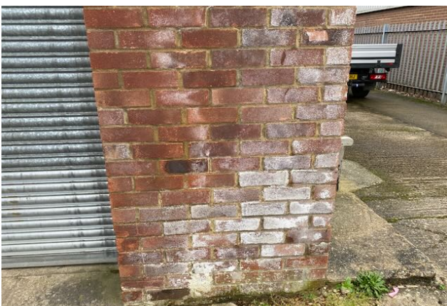
17: Efflorescence evident adjacent to roller shutter.
