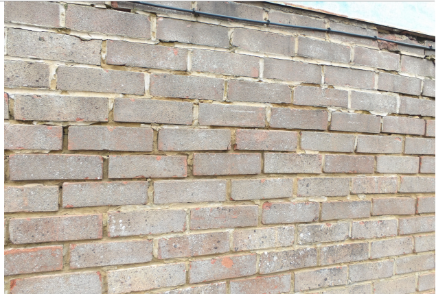
14: Previous repointing works are in poor condition.
