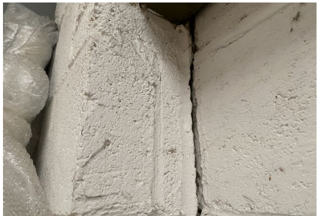
22. Failure of clockwork joints around steel frame.
