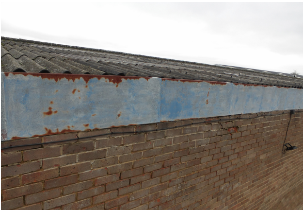
09: Corrosion to metal fascia sheets.
