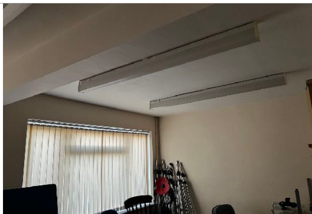
ME02 Office lighting in need of replacement.
