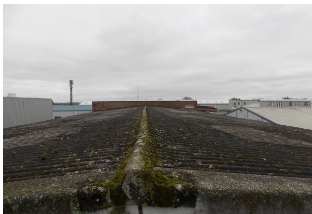
04: Moss build up to ridge of warehouse roof.
