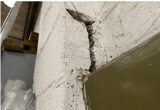
21. Failure of clockwork joints around steel frame.
