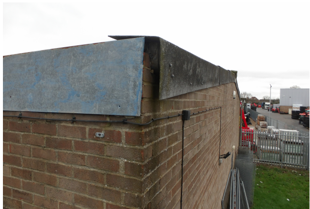
16: Saturated/stained brickwork due to failure in roof drainage.
