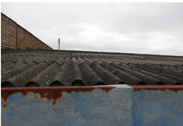
05: Corrosion to metal fascia sheets.
