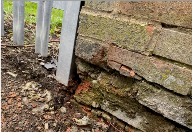
19. Spalled low level brickwork at rear of the warehouse.
