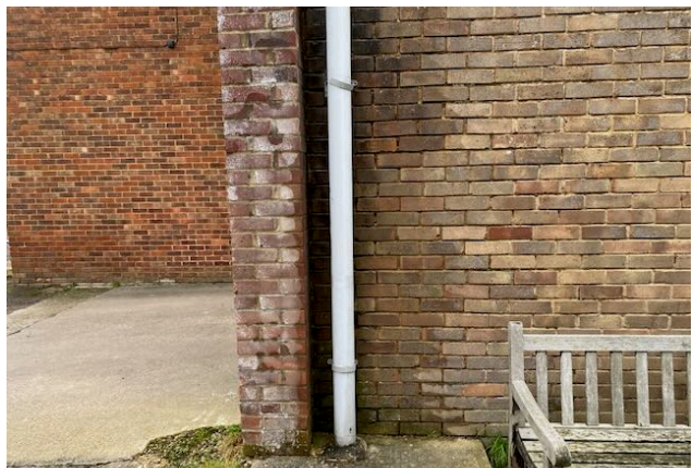
18: Failed rainwater outlet causing saturated brickwork.
