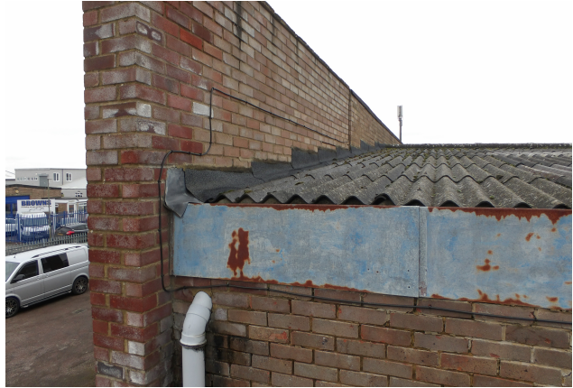
08: Failed downpipes and corroded metal fascia sheets.
