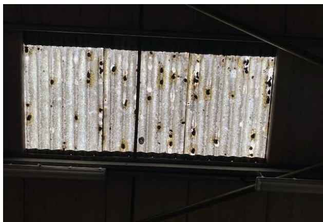
06: Discolouration and moss build up to rooflight above warehouse.
