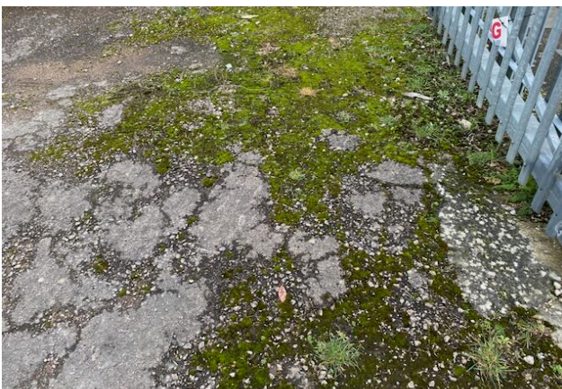
23. Tarmac parking space in poor condition.
