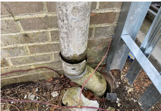
11: Failed downpipes in need of replacement (assumed ACM).
