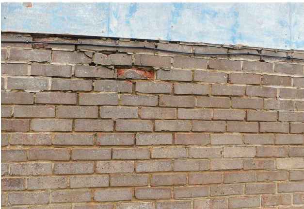
15: Spalling brickwork as a result of failed roof coverings.
