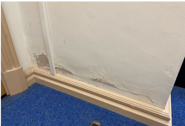
19. Delaminating paint to masonry wall in Reception.
