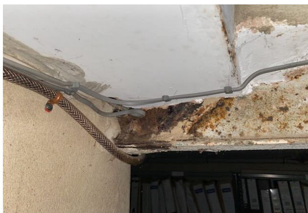
22. Corrosion evident to steel supports in basement.
