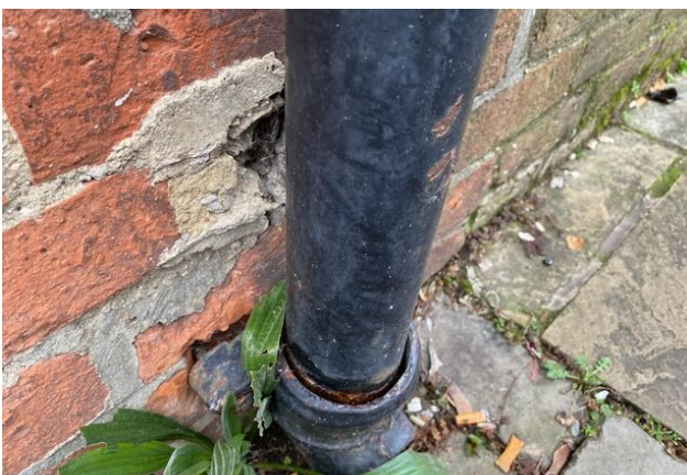
05. Vegetation growth and corrosion present at base of downpipe.
