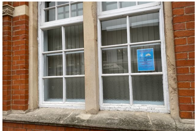
16. Spalled stone window reveals in need of repairs.
