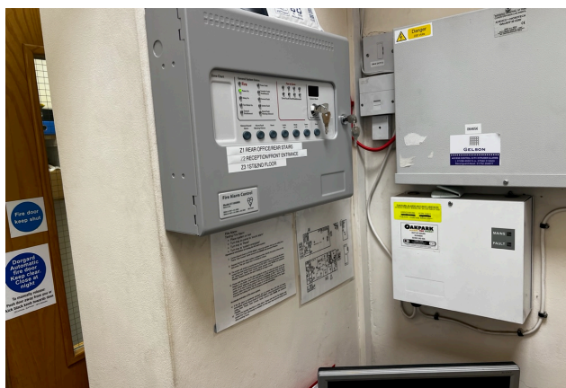
ME02. Fire alarm system approaching the end of life.
