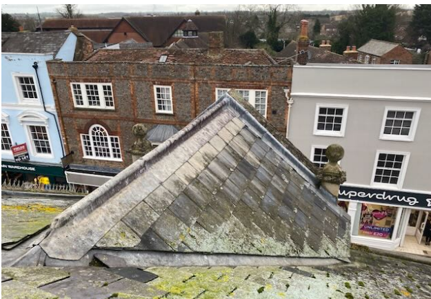
03. Moss, lichen and guano build up to slate roof coverings.
