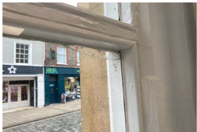
18. Crack in glazing on the ground floor.
