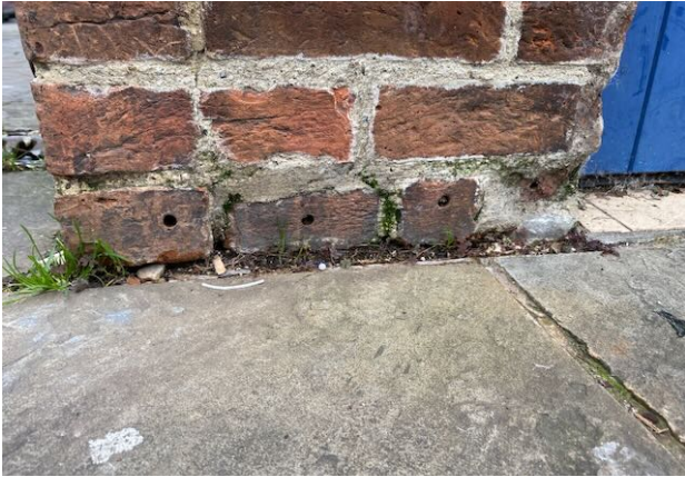
13. Evidence of previous damp proof injection works having been carried out.
