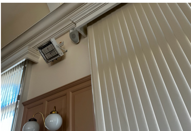
ME01. Electric radiant heaters due for replacement.
