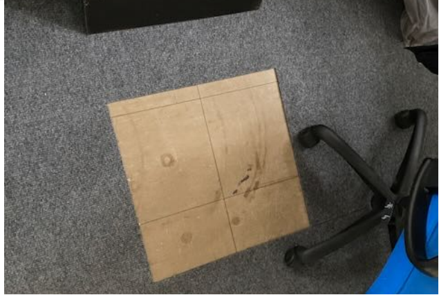
08. Missing Carpet tile to top floor office.
