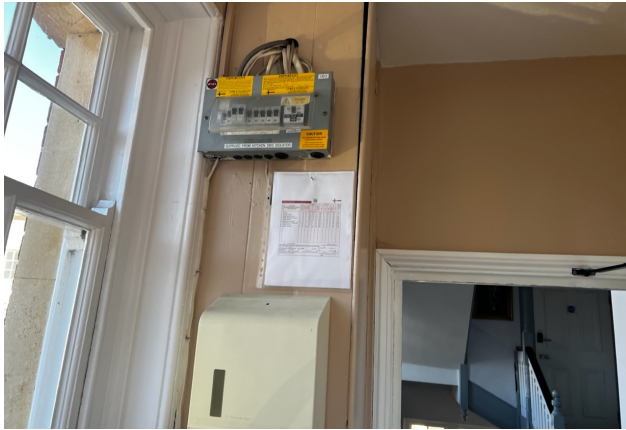
ME03. Distribution boards due replacement.
