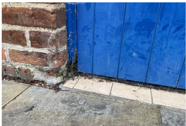
12. Rot present to external timber door frame.
