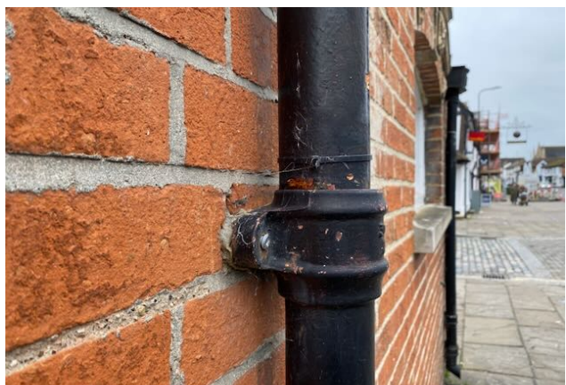
06. Corrosion present to downpipes.
