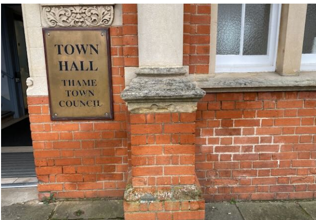
17. Evidence of saturated brickwork and stone detailing in need of repair.
