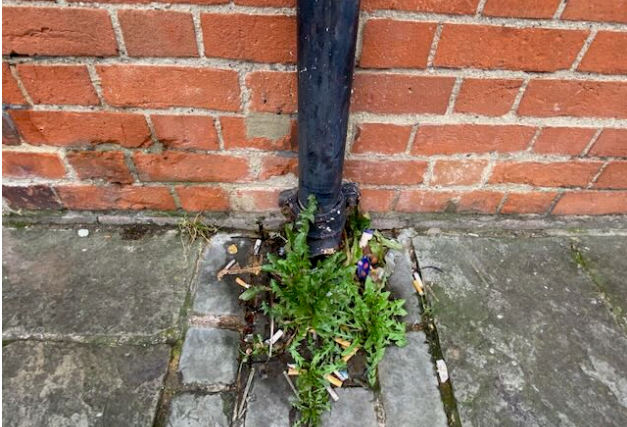
07. Vegetation preventing rainwater draining effectively.
