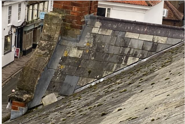
02. Slipped/dislodged tiles to dormer.
