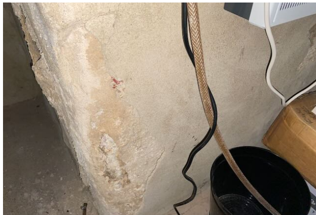
20. Delaminating render to basement
