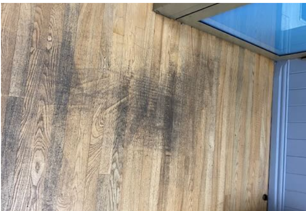
09. Worn flooring to Town Hall entrance.
