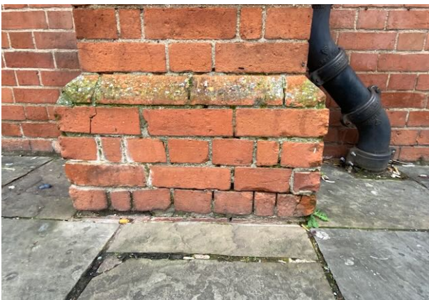
15. Loose/defective mortar jointing.
