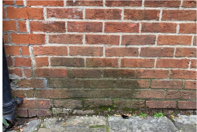
14. Evidence of saturated brickwork.
