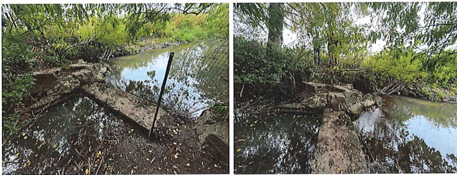
Figure 3 Photographs of the deteriorating weir structure
